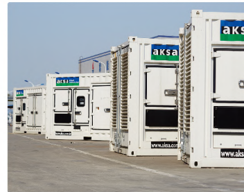
AKSA POWER GENERATION
